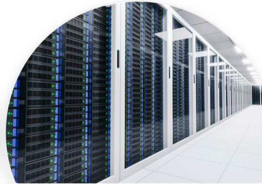
~64 racks per cluster
